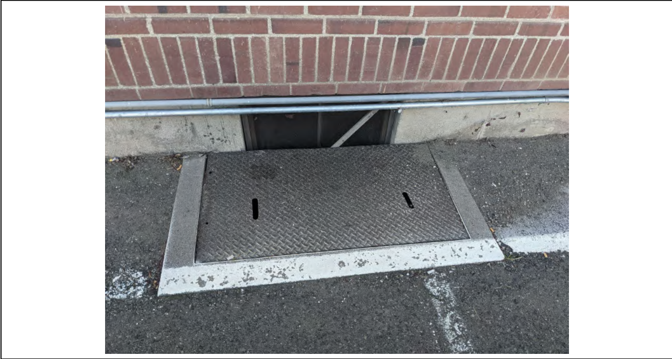
Elevation: B15585 Eastern lightwell on north wall of basement Photographer: S Rathbone
