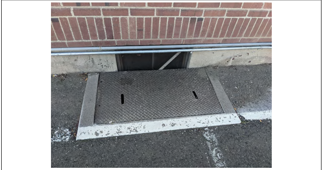
Elevation: B15585 Eastern lightwell on north wall of basement Photographer: S Rathbone
