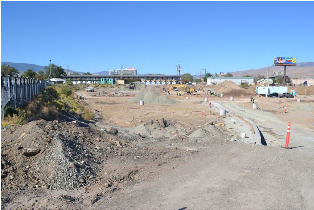
Elevation: Governor's Bowl Park construction site overview Direction facing: 260 Photographer: S Rathbone Date: 10/4/2022
