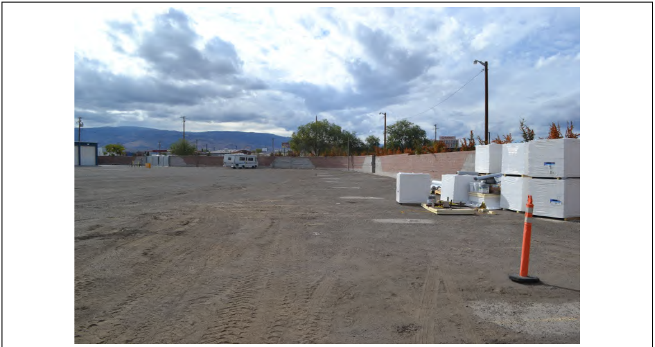
Elevation: Overview of CMU portion of Structure 2 Direction facing: 240 Photographer: S Rathbone Date: 10/25/2022
