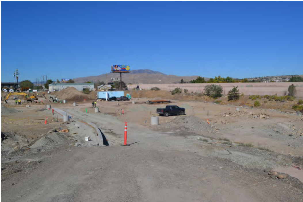
Elevation: Governor's Bowl Park construction site overview Direction facing: 310 Photographer: S Rathbone Date: 10/4/2022
