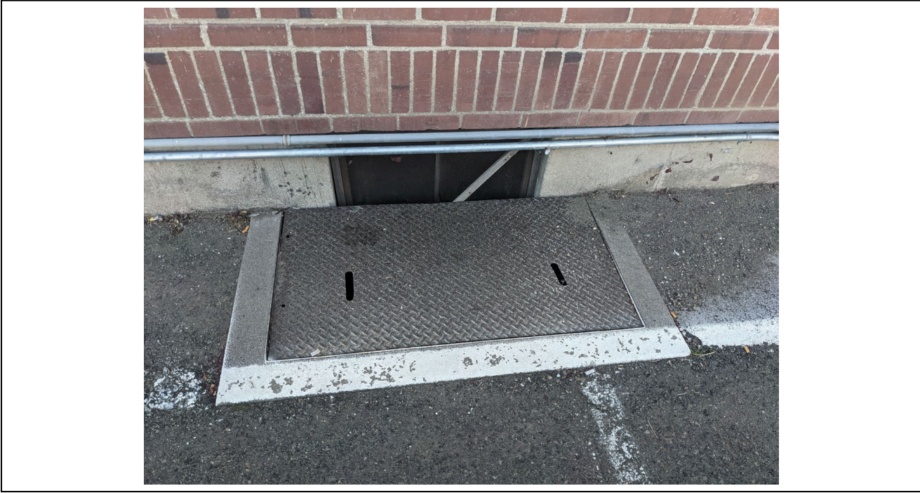
Elevation: B15585 Eastern lightwell on north wall of basement Photographer: S Rathbone
