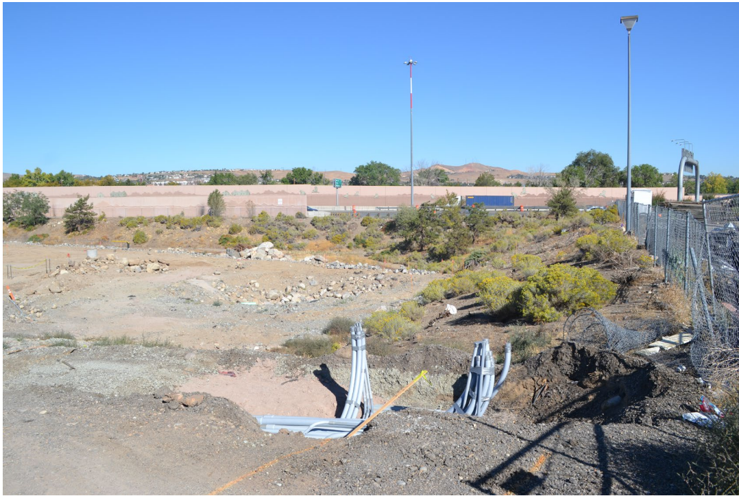
Elevation: Governor's Bowl Park construction site overview Direction facing: 350 Photographer: S Rathbone Date: 10/4/2022
