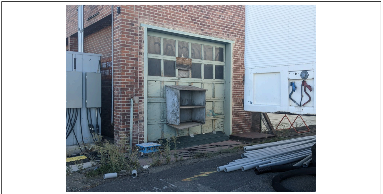
Elevation: Building 2 Door detail at east end of north wall Photographer: S Rathbone
