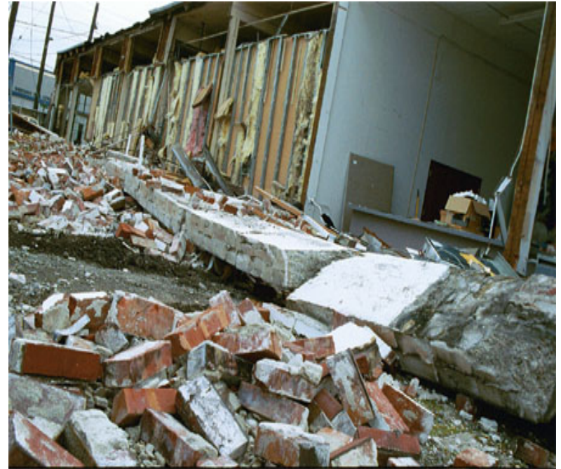
Seattle, WA, March 4, 2001 -- Scattered brick is all that remains of a First Ave. fabric store's wall.
