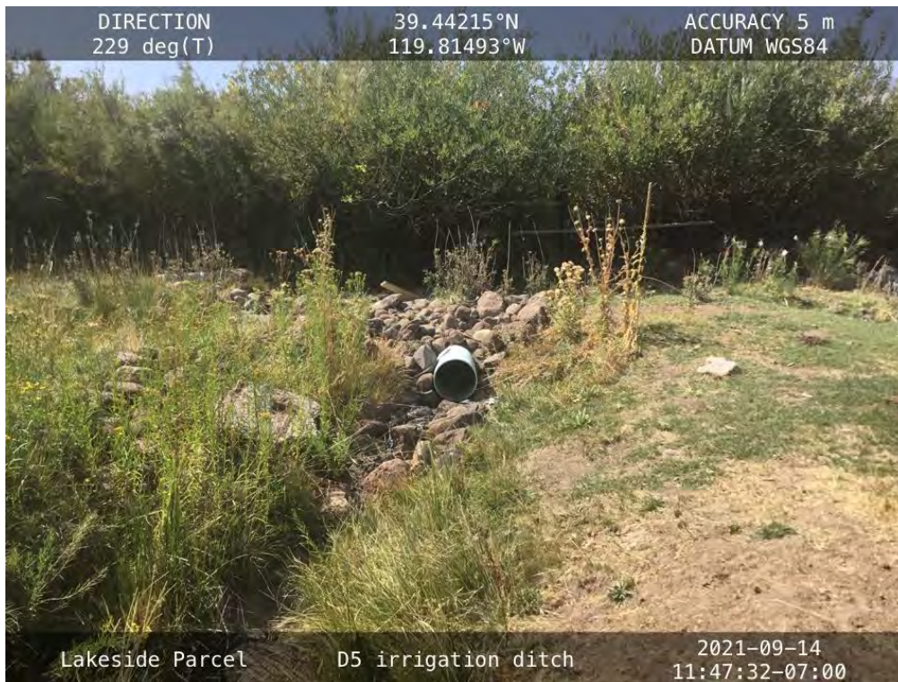
Photo 18. D-5: Irrigation ditch. Water from D-4 is discharged via a culvert under access road into D-5
