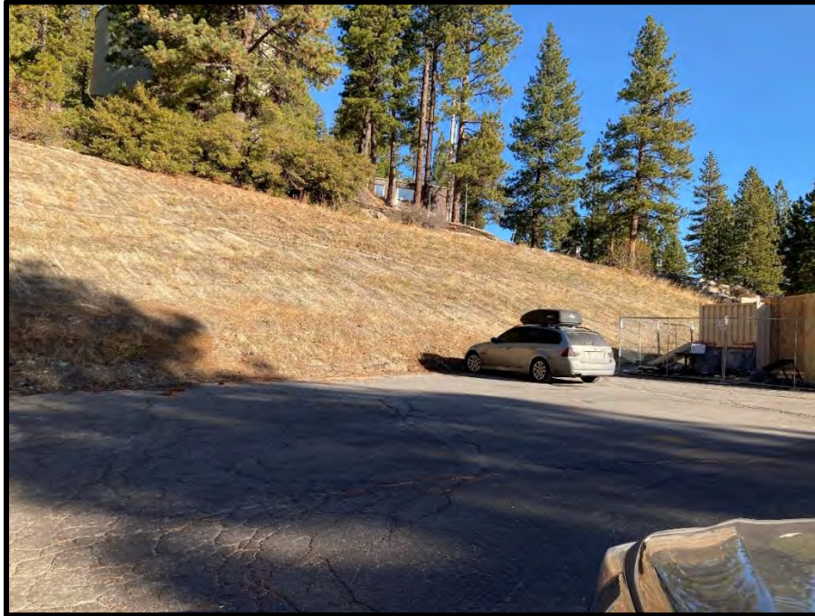
View of the existing slope at the northwestern corner of the site (terminus of Stateline Drive). At the top of the slope the current intersection of Reservoir Road and Lakeview Drive is situated. The photo is taken in the orientation of the approximate future alignment of the Lakeview/Stateline connector road.
