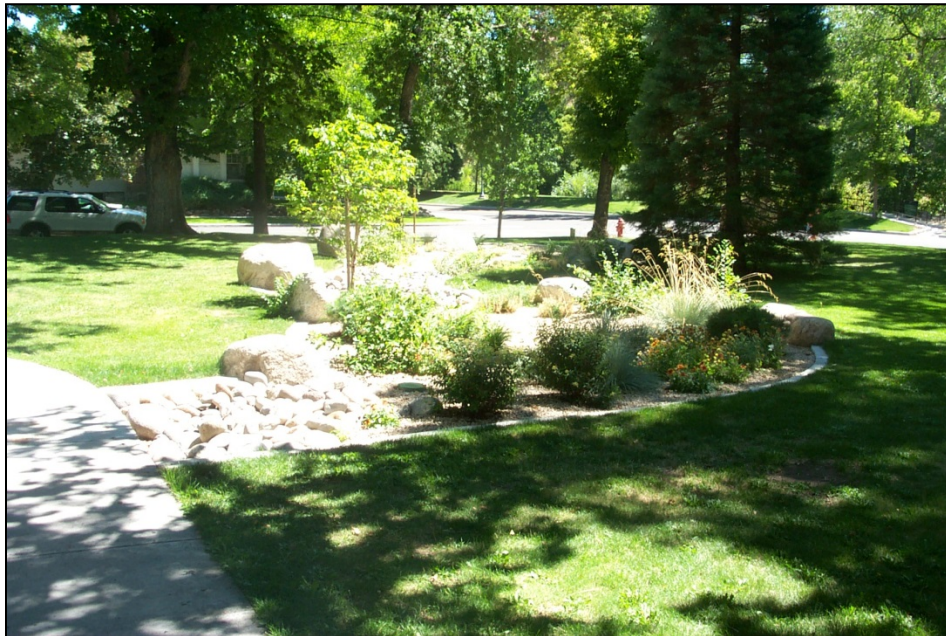
Figure 4-15. Rain Garden installed to collect and treat runoff from impervious surfaces at McKinley Arts Center. (Source: City of Reno)
