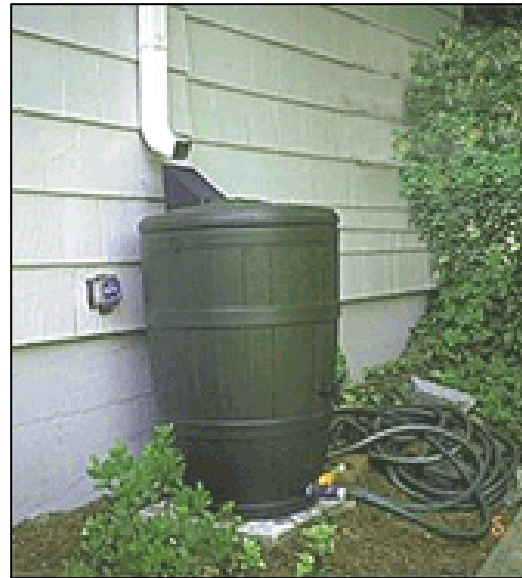
Figure 4-25. A typical rain barrel set-up at a residence. (Source: Low Impact Development Center)
