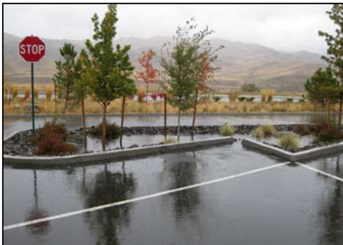
This parking lot island is designed to receive and infiltrate stormwater runoff from the parking lot. When the water-holding capacity of the island is exceeded, the water runs out the opposite side to a vegetated swale.
