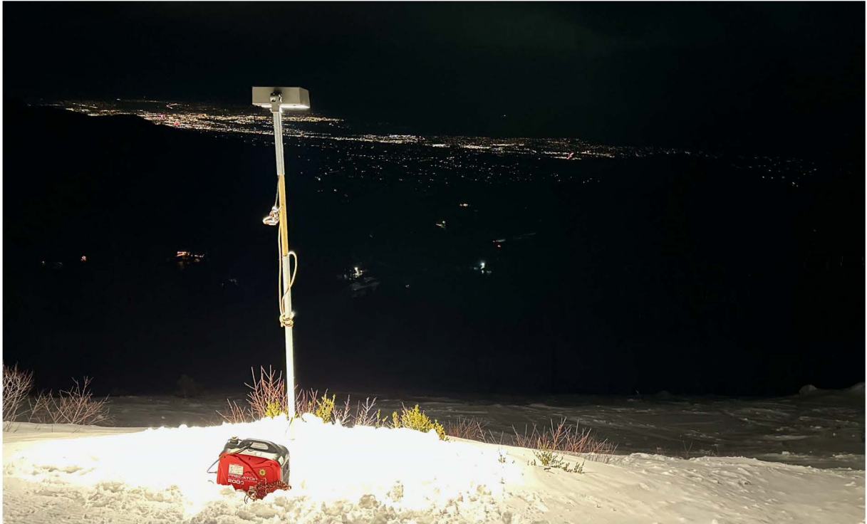
LOOKING EAST: ACTUAL FIXTURE INSTALLED AT CREST OF SKY TAVERN SKI AREA 2024-01-19
