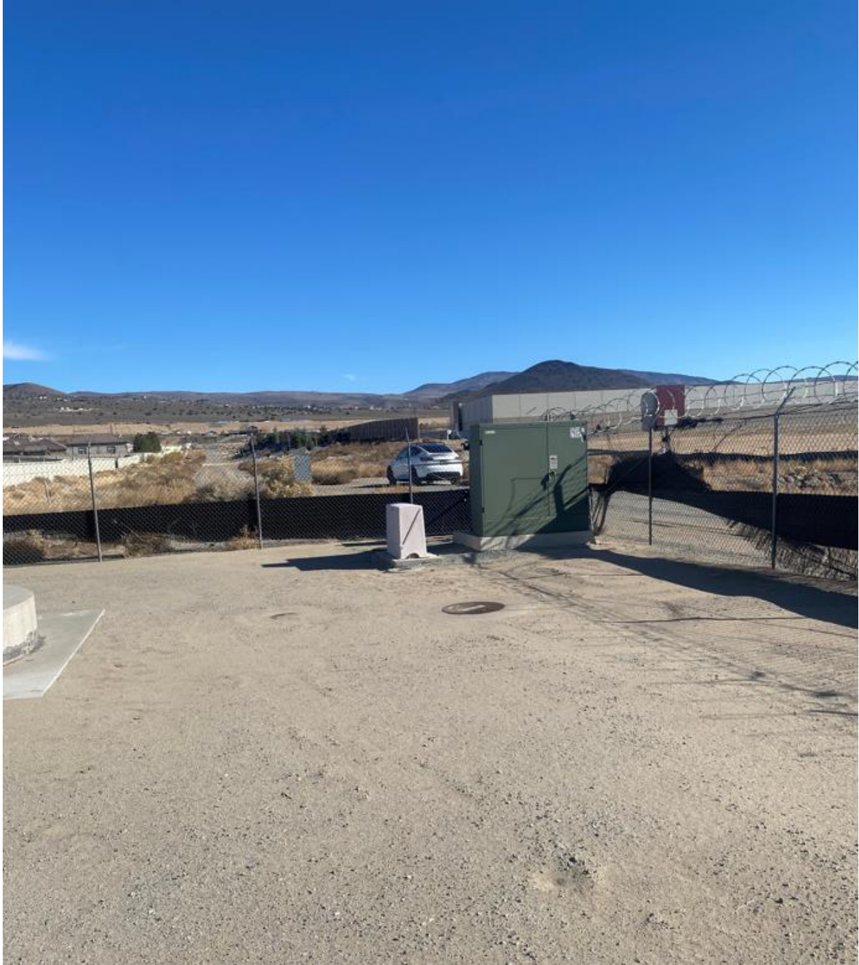
Figure 9: Example of a Similar Use Washoe County Sewer Lift Station in Spanish Springs
