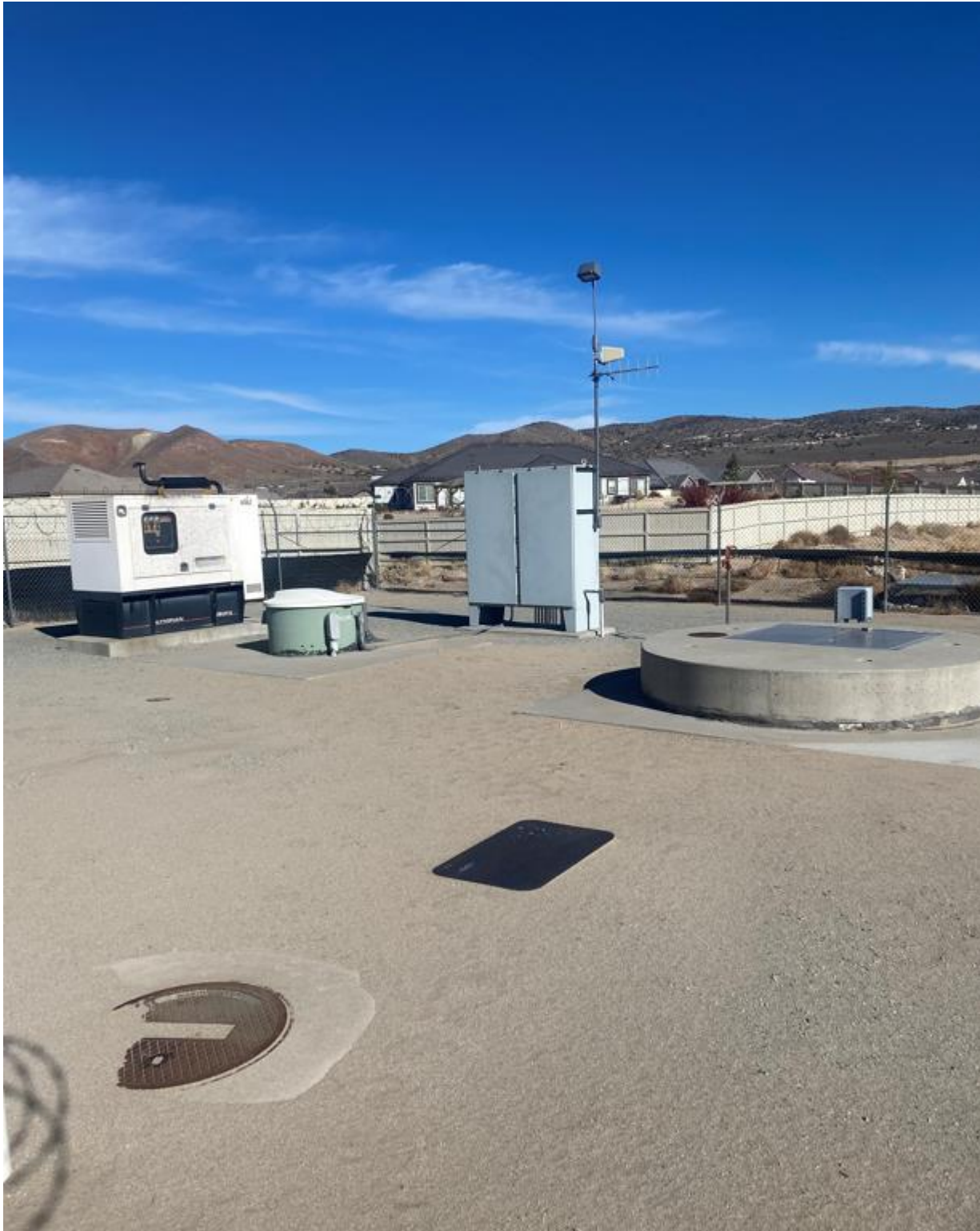
Figure 9: Example of a Similar Use Washoe County Sewer Lift Station, cont.
