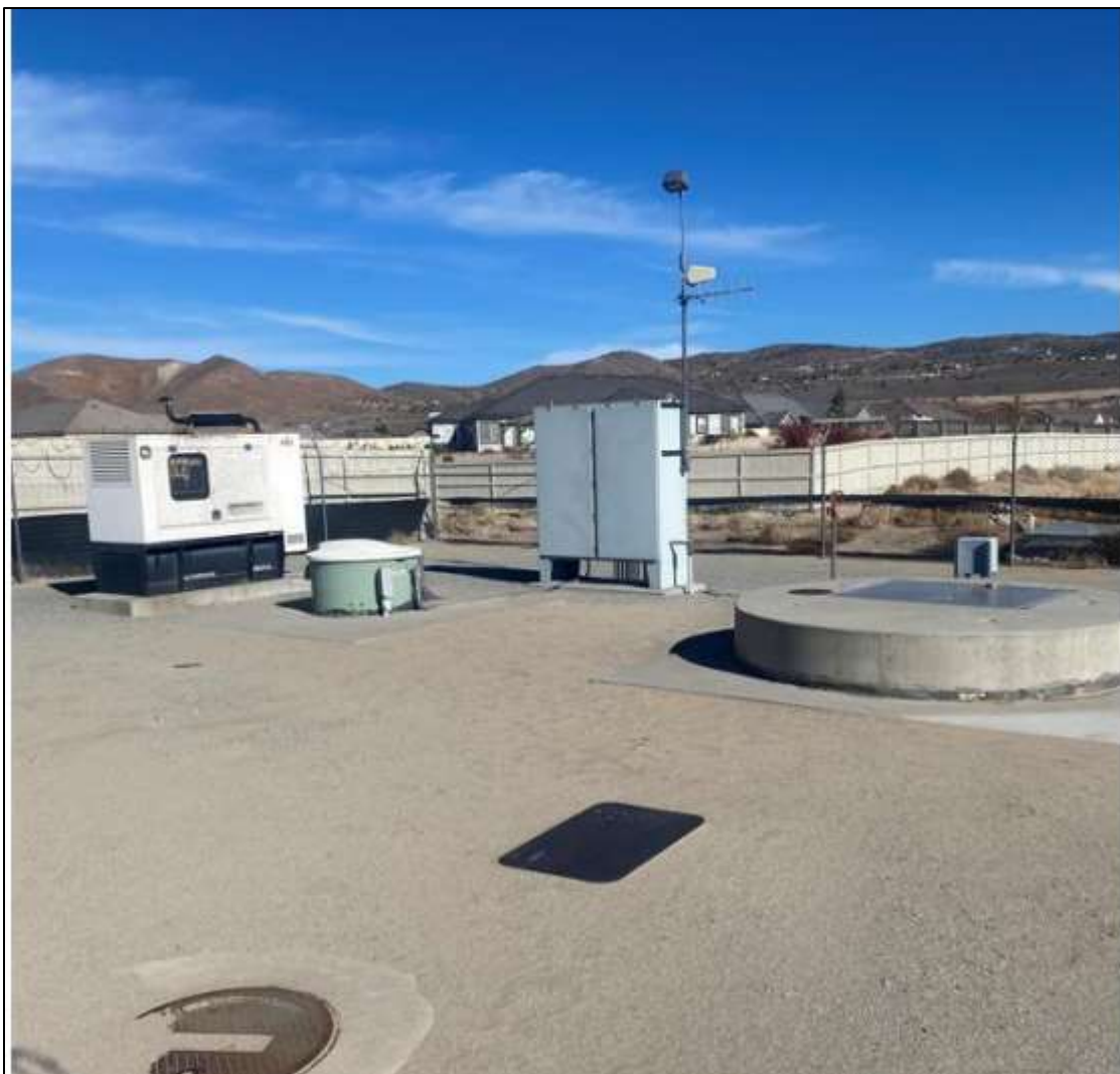
Example of Similar Use – Spanish Springs Sewer Lift Station
