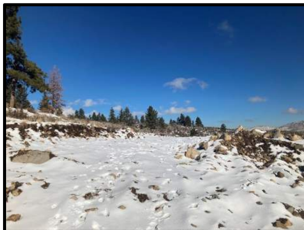
View to the north of unpermitted grading at the northwestern corner of the site.
