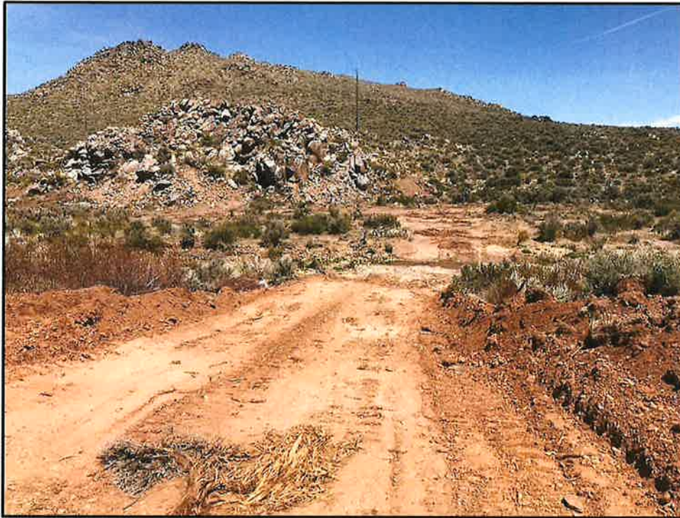
Portion of new access that was "graded" to get across a steep slope on west side of drainageway.
