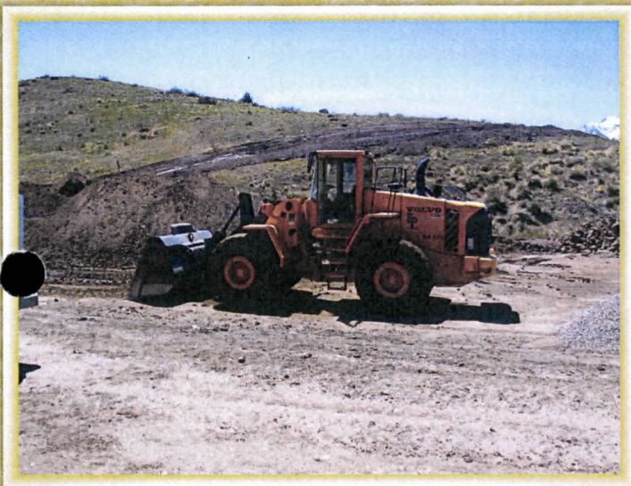
These photos depict FP Construction equipment and wetted area around dirt piles. This water dumped by loading water in scoop of front loader from pond in area. 4-29-09.
