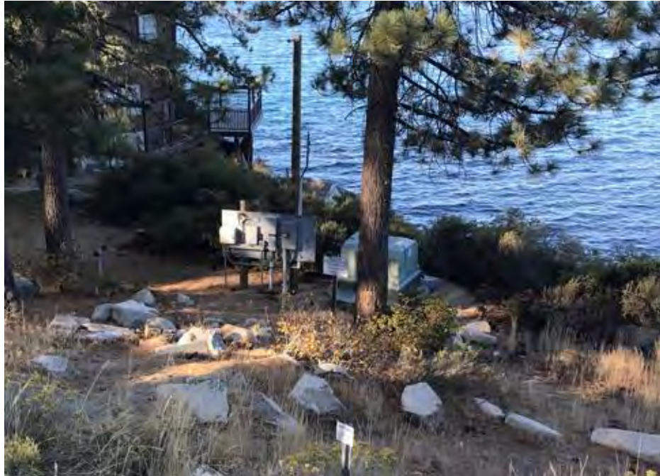
Incline Village GID Lift Station
