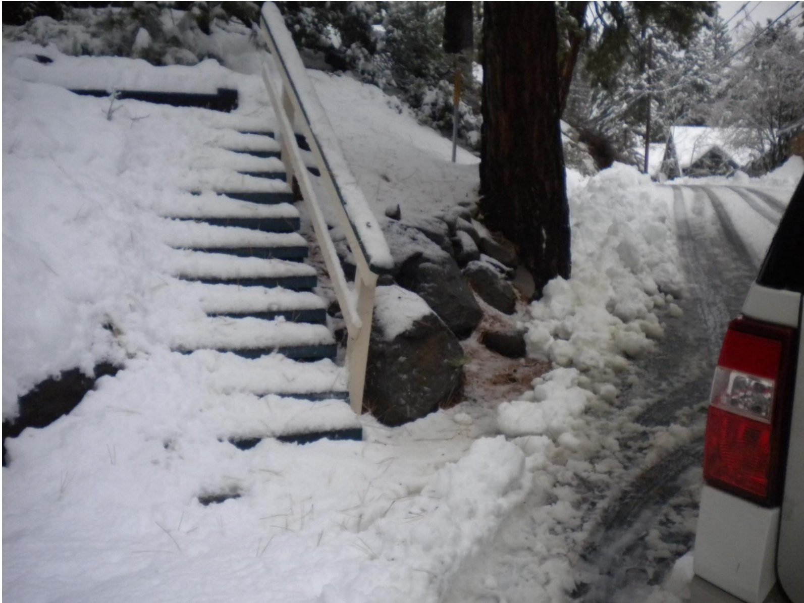
Picture #5 – looking north on Tuscarora rd. showing stair case, large boulders and tree that are across the street and directly in line with the garage door opening.
